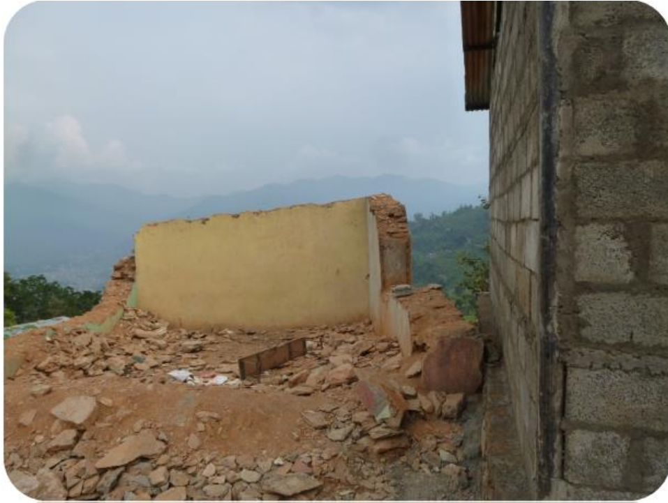
Damaged Shree Kalika Primary School, Nilkantha, Dhading
