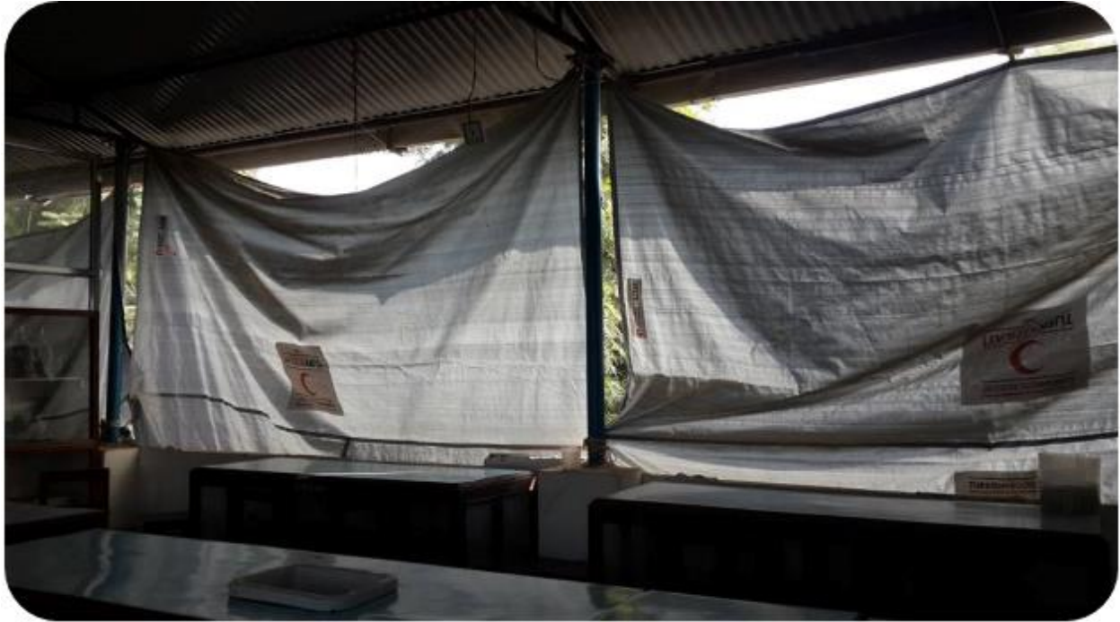
Damaged lab at Shree Padma Higher Secondary School, Bhaktapur
